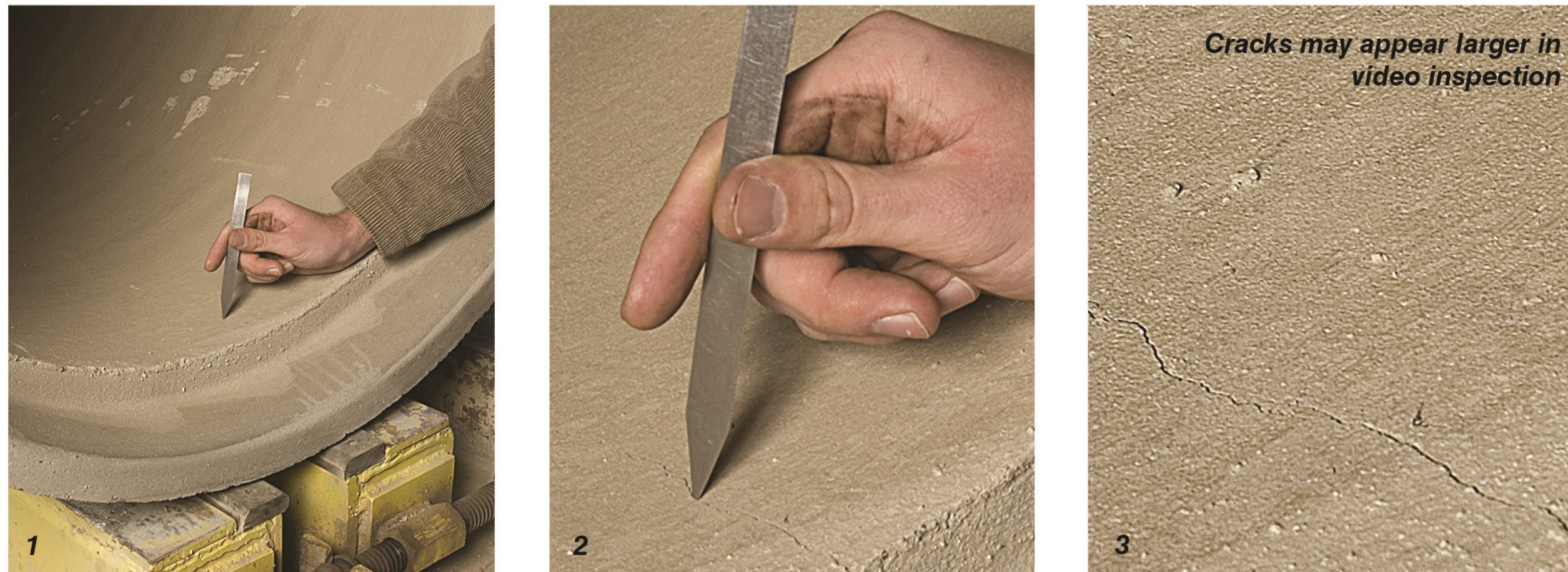
0.01-Inch Crack Measured in a 36-Inch, Class IV Pipe. Pictures 1, 2, and 3 shown as if viewing the crack standing, kneeling, or through a video inspection, respectively.
